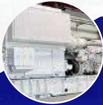
Genset with IP55 CACA Generator
