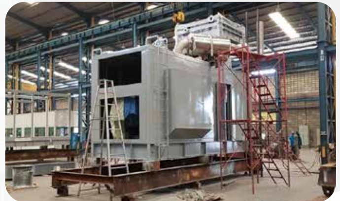
Genset Assembly Area
