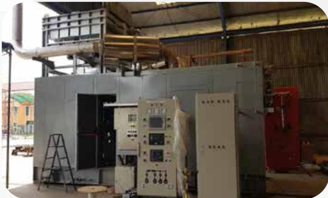
Genset Testing Area
