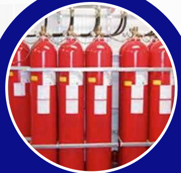
CO2 Fire Suppression System
